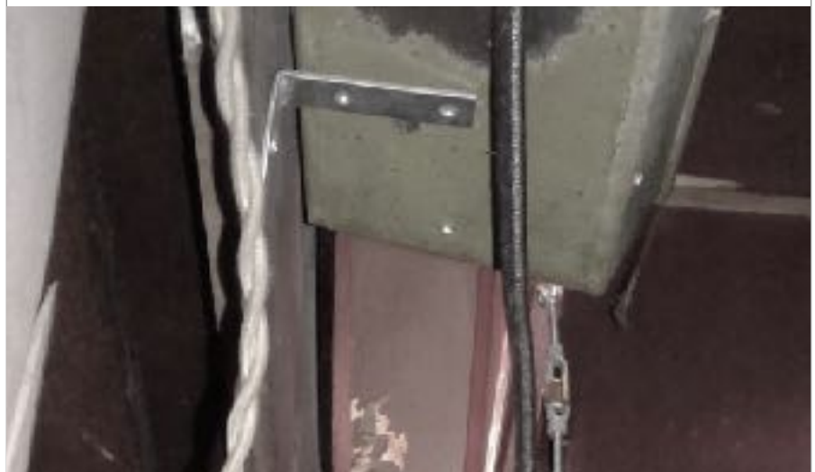
Behind the High Altar showing the aging wiring and old loaf pan reflector.
